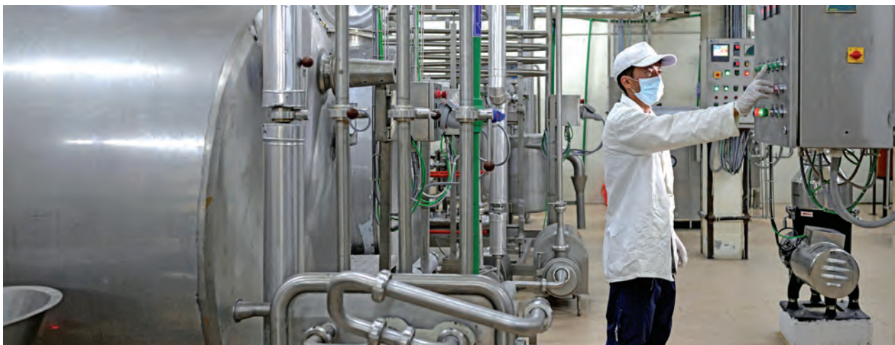
Milk Processing Plant, Ladakh
